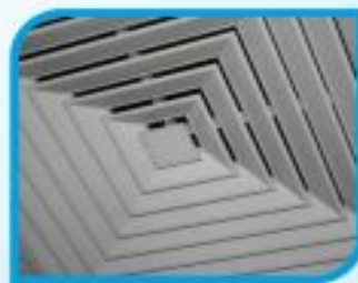
Ac Ducting Diffuser/Diffuser
