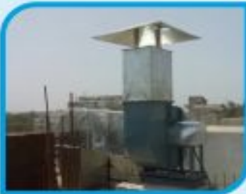
Kitchen Exhaust Blower
