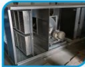
Clean Room Air Handling Unit
