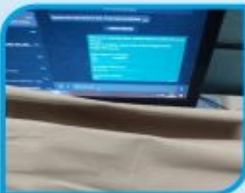
Fire Rated duct Canvas Connection
