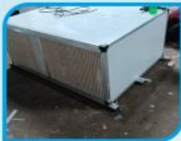
Ceiling Suspended Air Handling Unit
