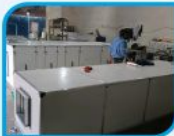
Air Handling Unit
