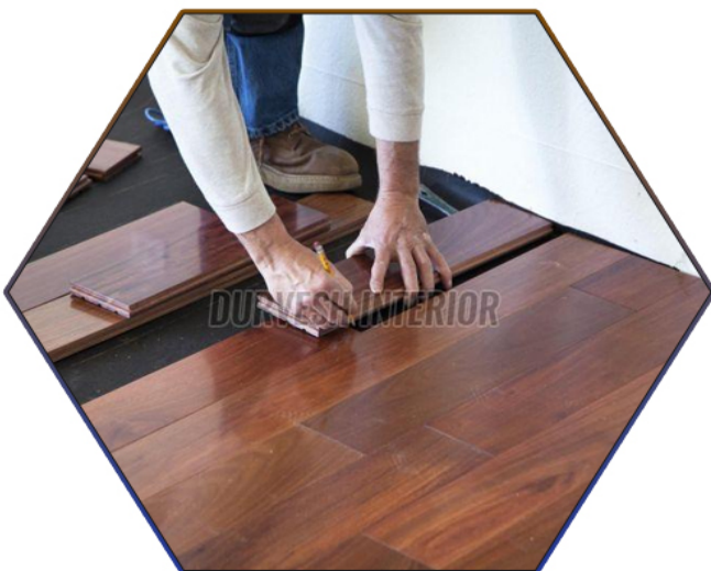
LAMINATED WOODEN FLOORINGS
