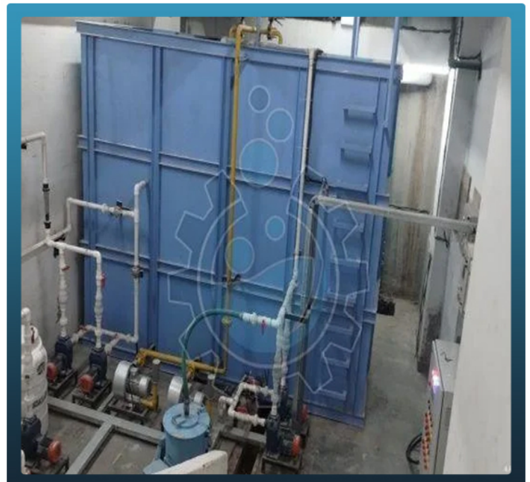
MBR Based Sewage Treatment Plant
