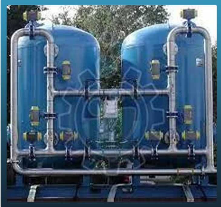
Automatic Industrial Water Treatment Plant
