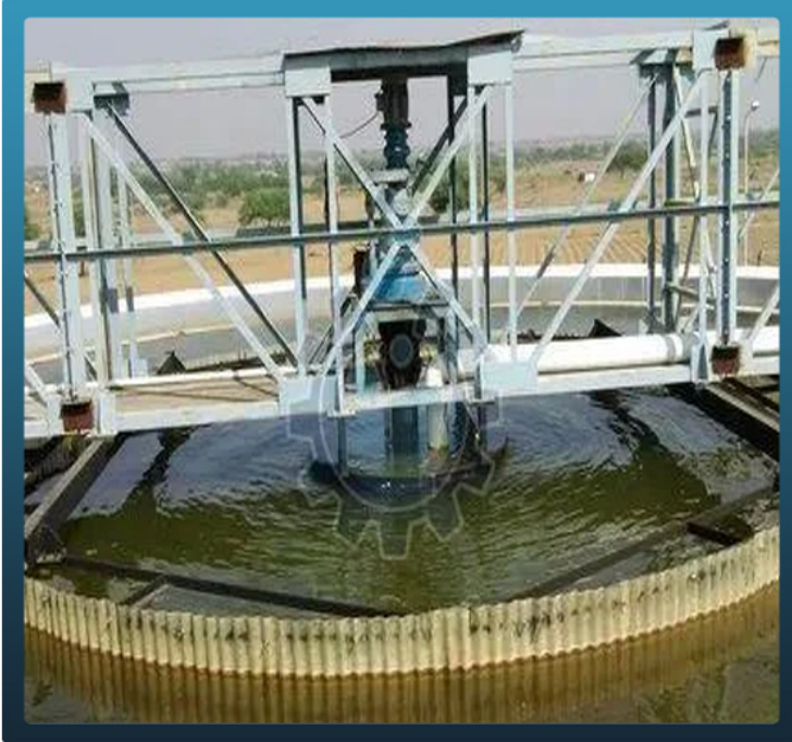
High Rate Solid Contact Clarifier
