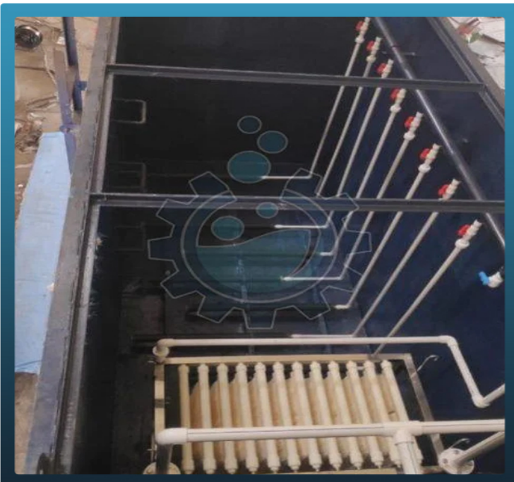
Membrane Sewage Treatment Plant
