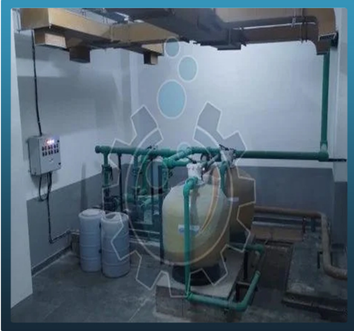
Swimming Pool Filtration Plant
