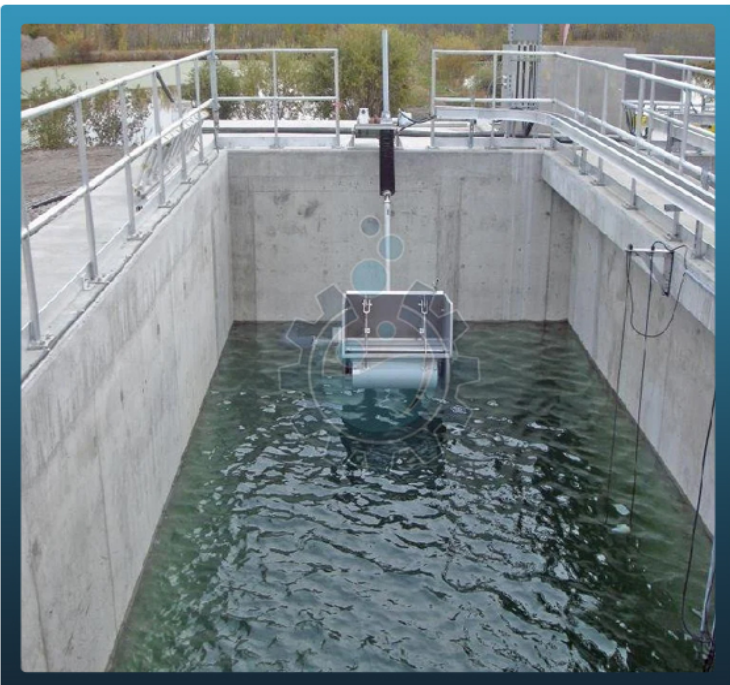
SBR Sewage Treatment Plant
