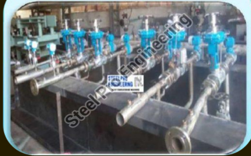
Spray Cooling Piping System
