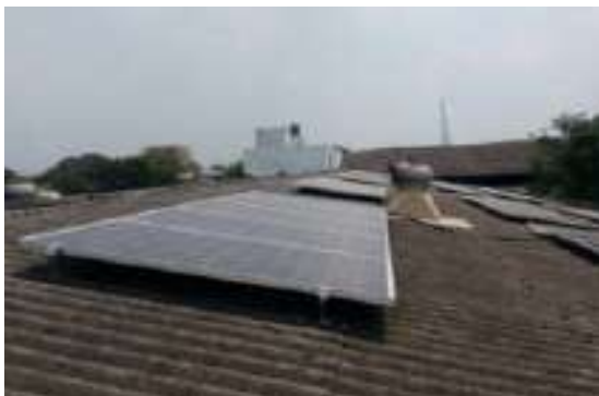
250 KW ALLIED ELECTRICAL, VADODARA
