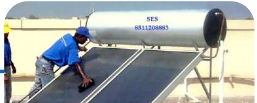
Solar Water Heater
