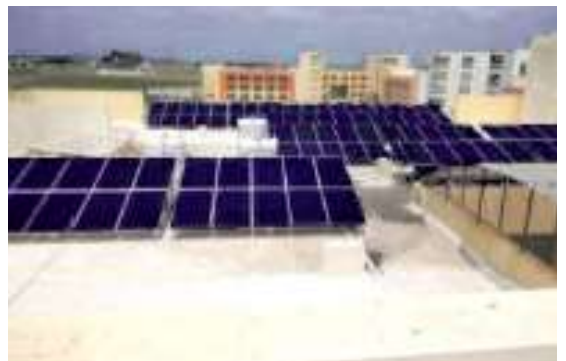
290 KW COLLECTOR OFFICE, KHAMBHALIA
