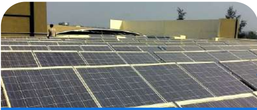
Solar Rooftop Systems
