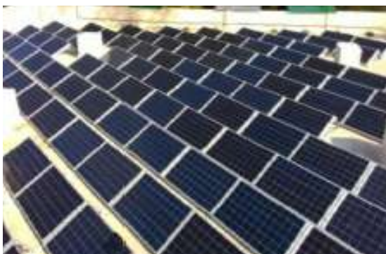
520 KW CIVIL HOSPITAL, DHARAMPUR
