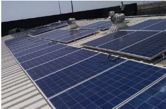
145 KW NEXA SHOWROOM VADODARA
