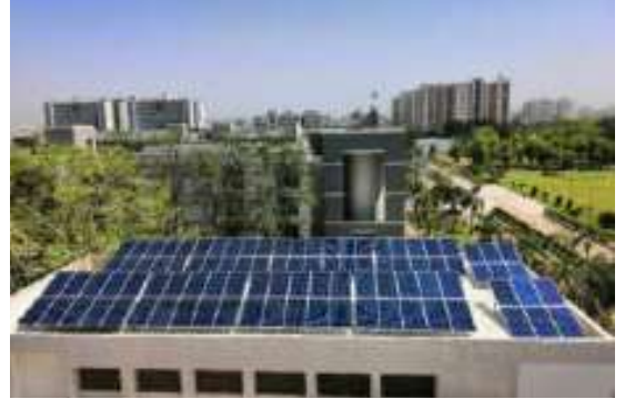
15 KW GUJARAT COURT, AHMEDABAD
