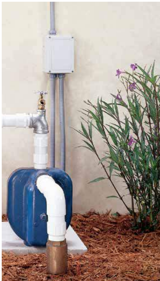
pump start relays
