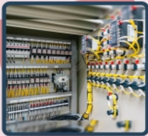
Control Panel Wire Harness
