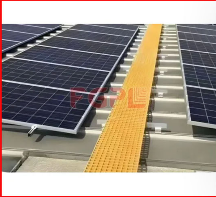
FRP Rooftop Walkway
