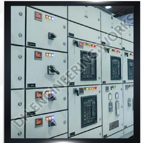
Low Voltage Panels
