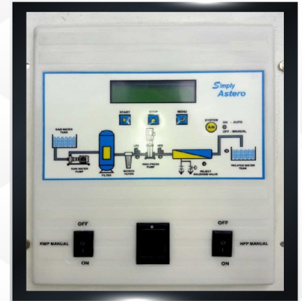
Ro Control Panel
