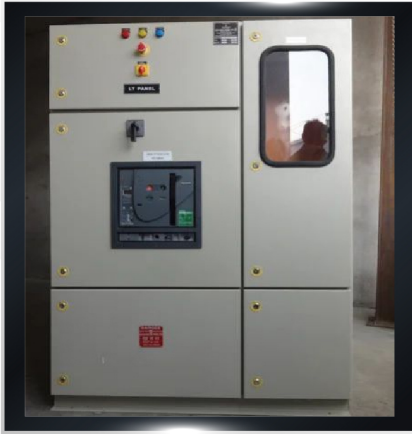
ACB Distribution Panel
