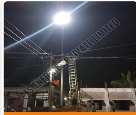
Aluminum Street Light Pole
