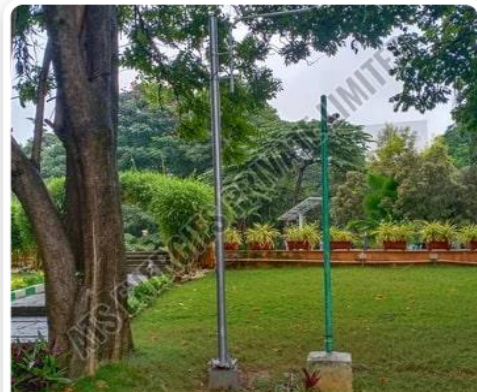
Tubular CCTV Camera Pole
