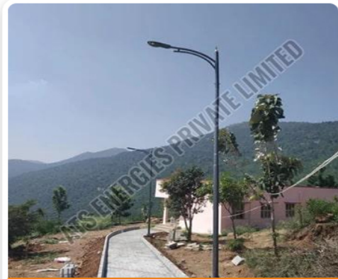
Round Galvanized Iron Pole
