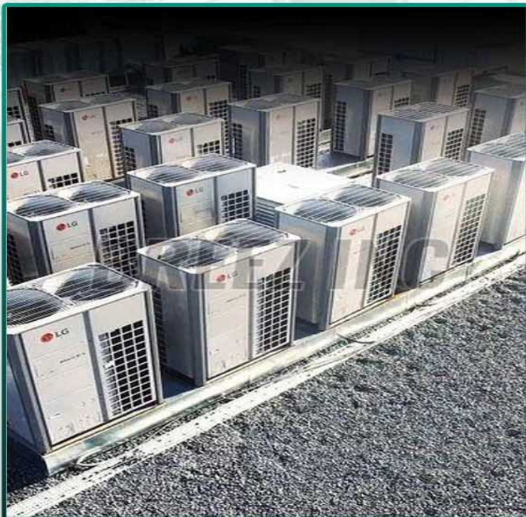
VRF Air Conditioning System
