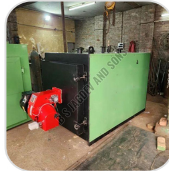
Diesel Fired Steam Boiler
