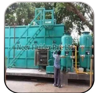
SBR Sewage Treatment Plant
