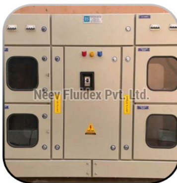
Three Phase Meter Distribution Control Panel
