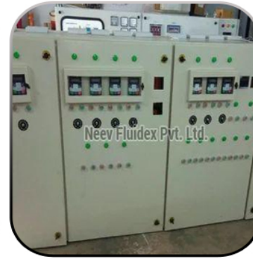
440 V MS Electric Control Panel
