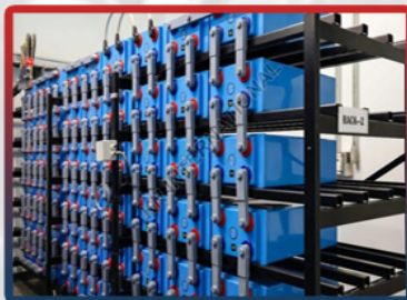
Electrical Battery Charging Unit
