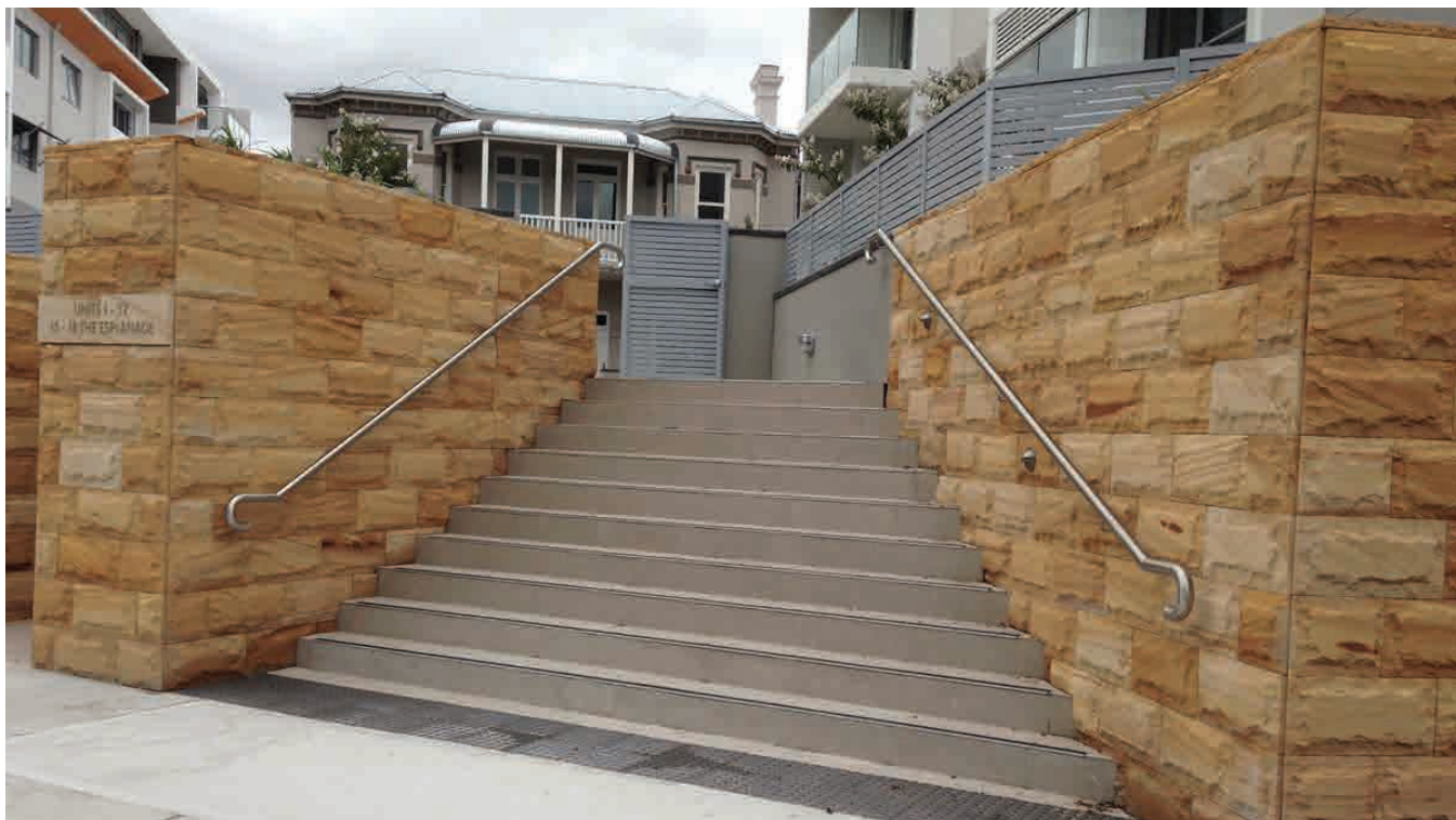
SANDBLASTED CHIPPED EDGES
