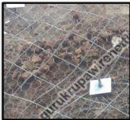
Rock Fall Protection System
