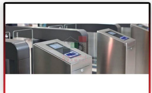
Turnstile Access Control System
