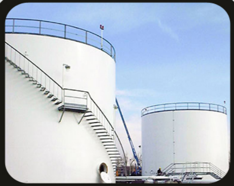
Aviation Fuel Storage Tank
