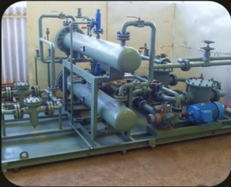
Fuel Handling System
