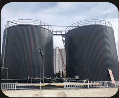
Bitumen Storage Tank
