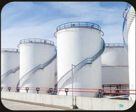
Petroleum Storage Tank
