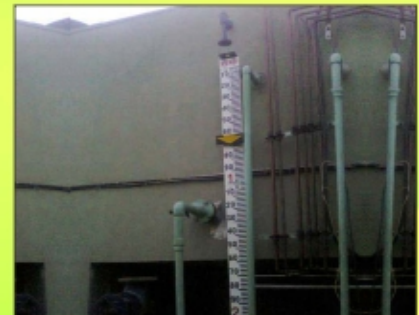
007 Float & Chord Level Gauges
