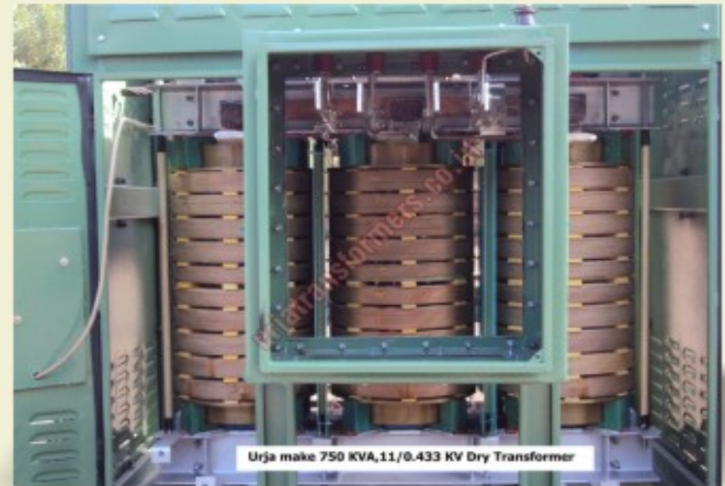
Dry Transformer VPI 02
