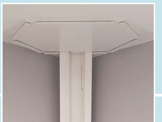
Fire seals for both lower and upper floor lift use
