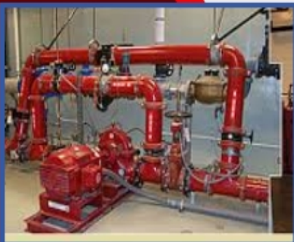
Fire Fighting System
