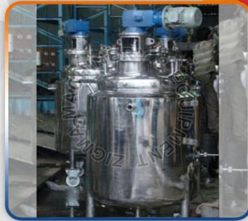
Cocoa Processing Plant
