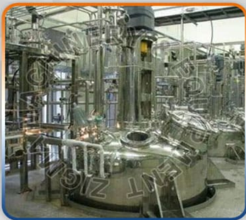
Ointment Paste Processing Plant
