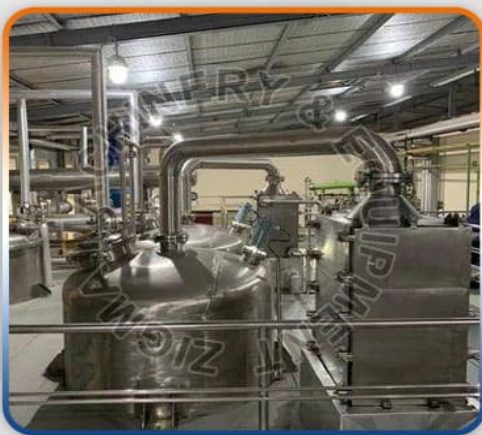
Curcumin Oil Processing Plant
