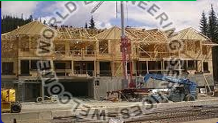
Residential Electrical Work Services
