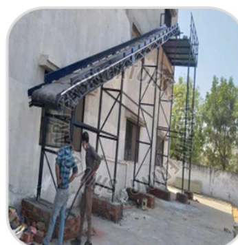
Rubber Belt Conveyor System
