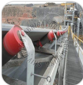
Inclined Belt Conveyor System
