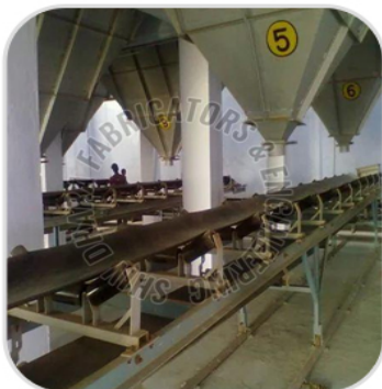
Hopper Feeding Conveyor System
