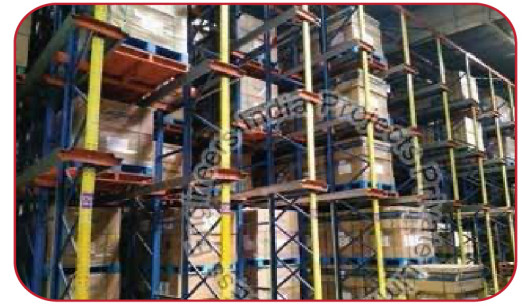
Drive Pallet Racking System
