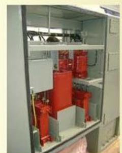
AC Loco Panel
