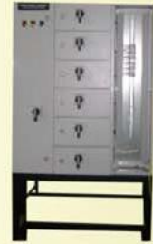
Power Distribution Panel
