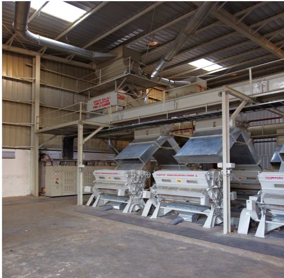
Twin Auto Regulator Individual Gin Feeding Conveyor System
