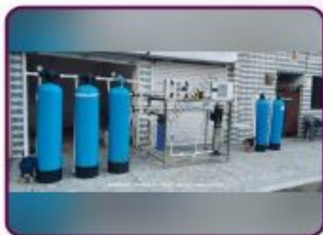
Reverse Osmosis Plant
