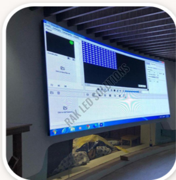
Auditorium LED P2.5 Indoor Display Screen
