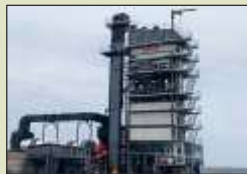
ASPHALT BATCH PLANT
