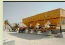
WET MIX PLANT
