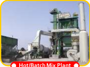
Hot/Batch Mix Plant
