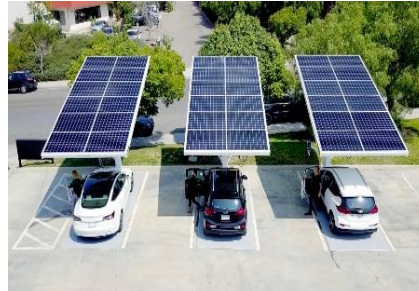
Solar Tree EV Charger
