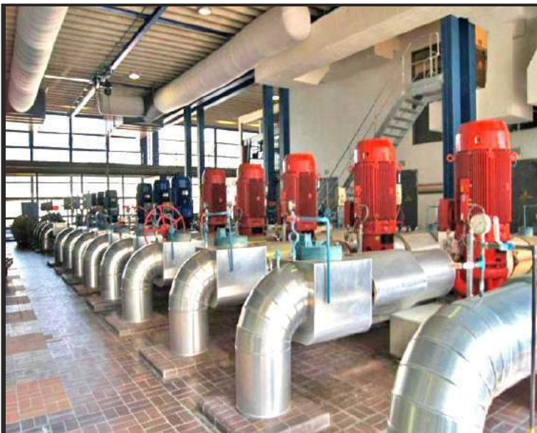
IN-LINE PUMPS WORKING AT A.C PLANTS
