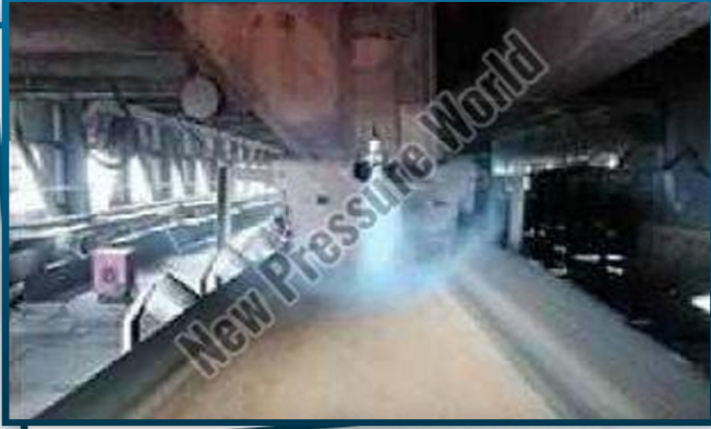
Dust Suppression System
