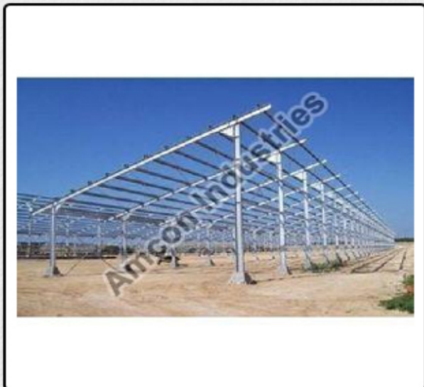
Steel Solar Panel Structure
