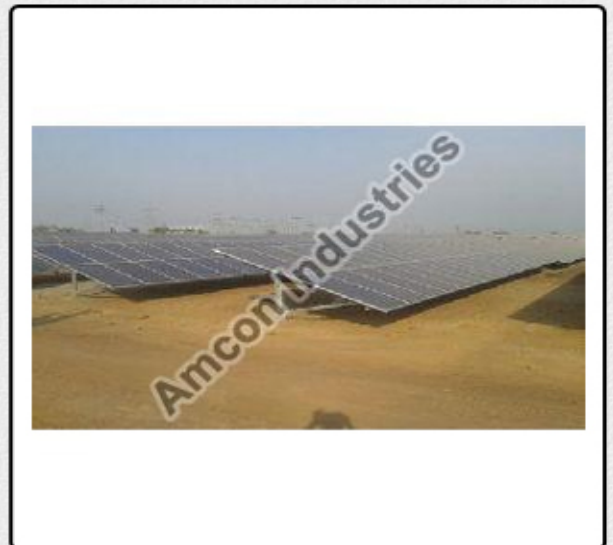
Mild Steel Solar Panel Structure
