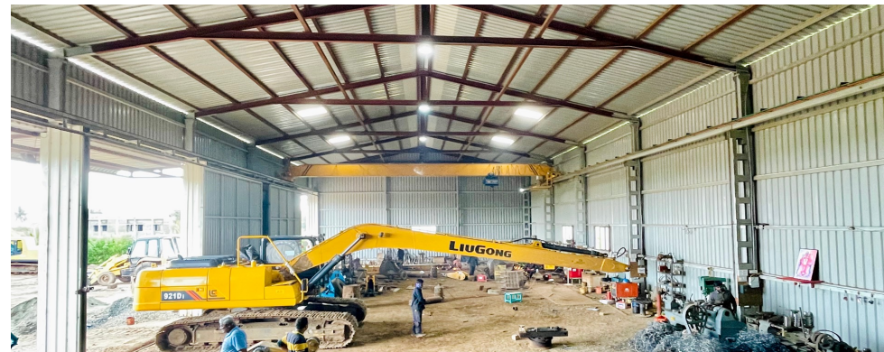
ii. Overhead Crane 8 Ton Capacity
