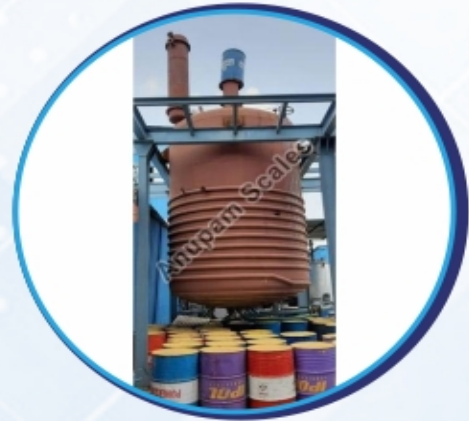
ELECTRONIC TANK WEIGHING SYSTEM
