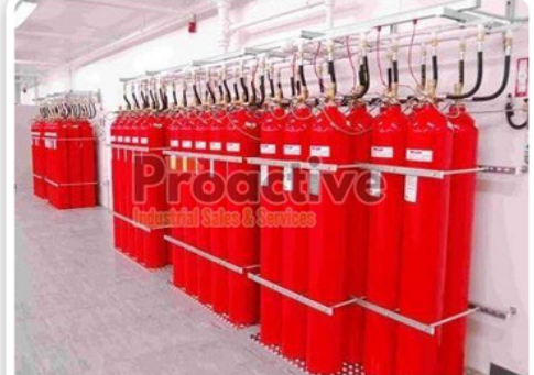
Fire Suppression System
