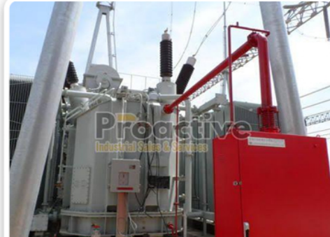
Nitrogen Injection Fire Protection System
