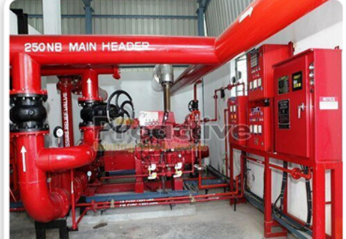
Fire Hydrant Pump System
