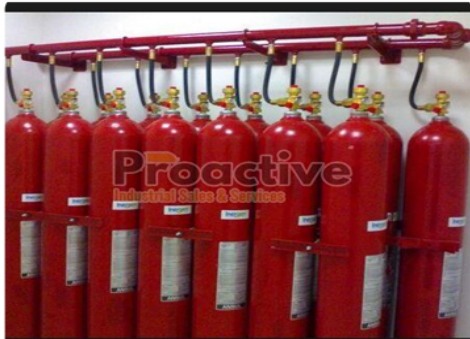
Co2 Flooding System
