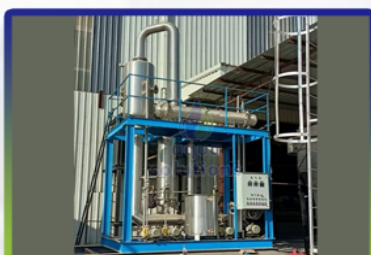
Multi Effect Evaporation Plant
