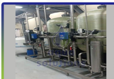
Water Filtration Plant
