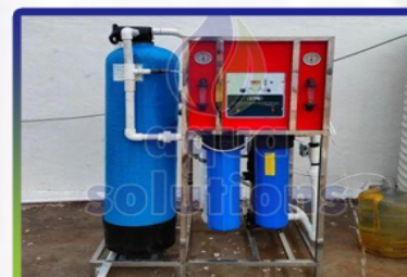
Semi Automatic DM Water Plant
