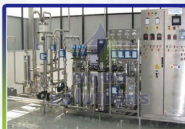
Purified Water Generation System
