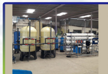
Reverse Osmosis System
