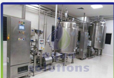
Purified Water Distribution System
