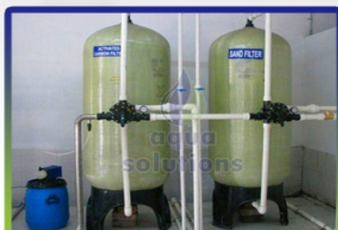
Pressure Sand Filters
