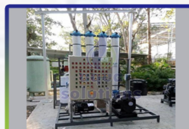
Industrial Ultrafiltration Plant
