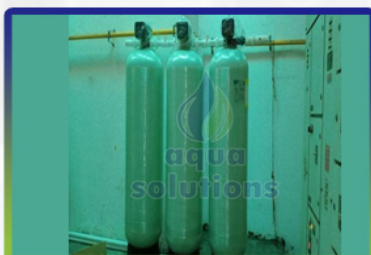
Water Softener System
