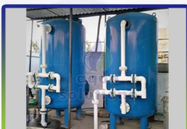
Water Purification System
