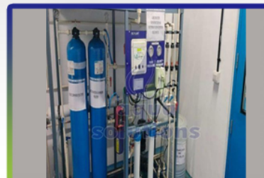
Commercial RO Water Purification Plant
