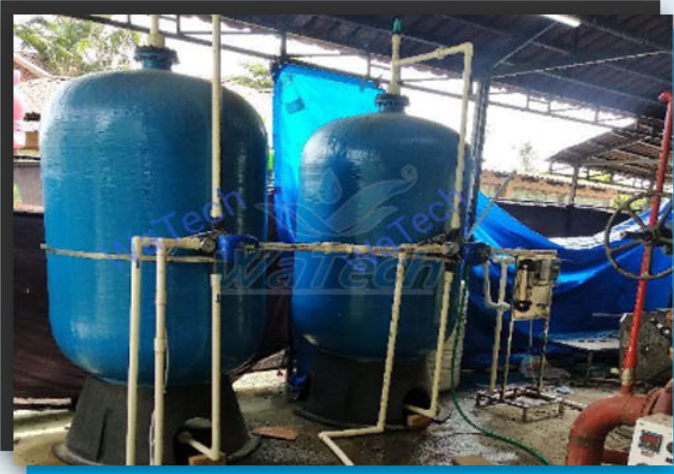
Industrial Water Softener
