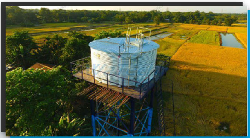
Zinc Aluminium Water Tank
