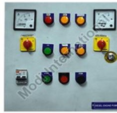
Direct Online Starter Control Panel
