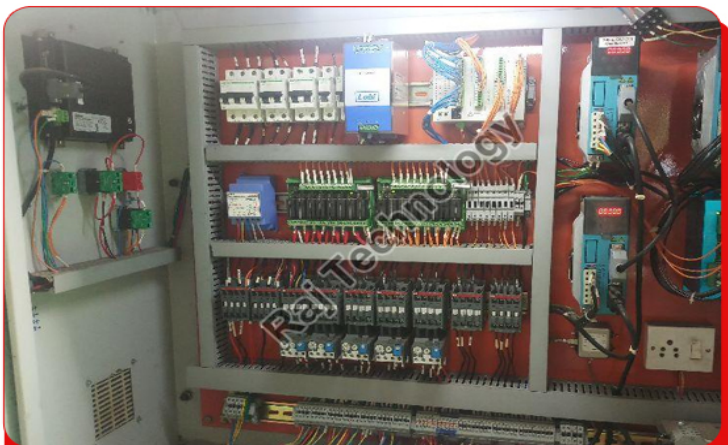
Electrical Control Panel
