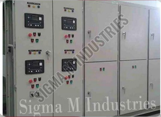
Electrical LT Distribution Control Panel
