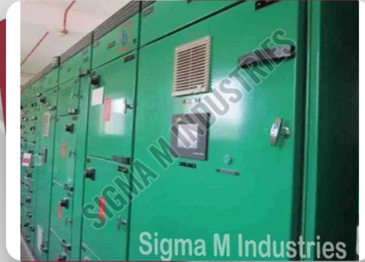
MDB Control Panel Board
