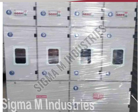
EB Metering PCC Panel
