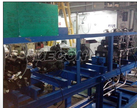
Hydraulic Power Packs & Valve Stand
