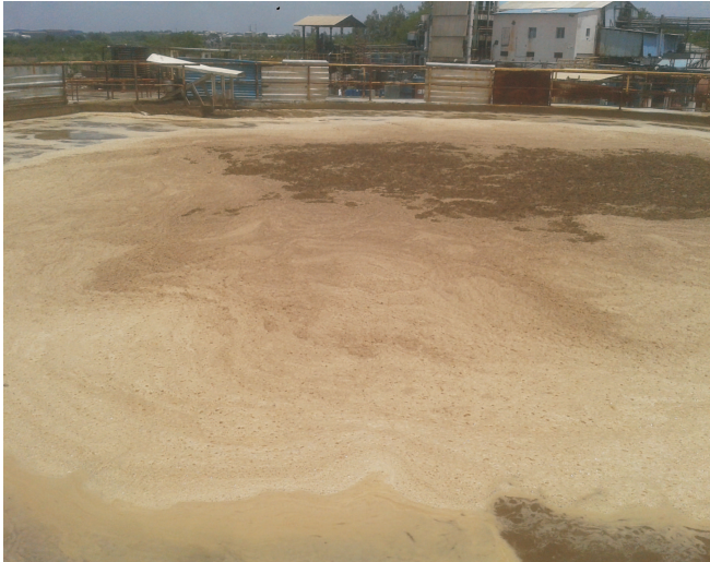
Aeration Tank - Before start of biological treatment there was thick layer of sludge floating on the surface of aeration tank 1st.
