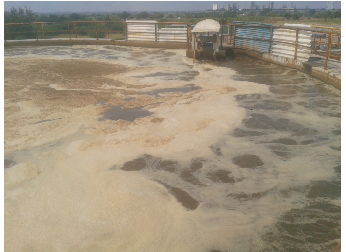
Aeration Tank 1st - After Biological treatment, there was good reduction in sludge layer after 6 weeks of biological treatment.
