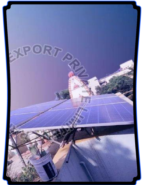
On Grid Solar Rooftop System
