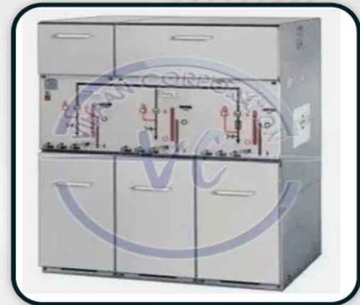
Siemens Ring Main Unit
