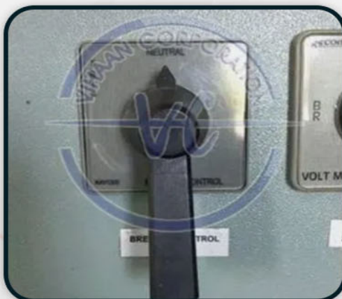
Local Remote Selector Switch
