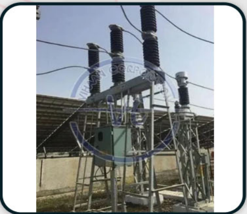
66 Kv ABB Hitachi SF6 Circuit Breaker
