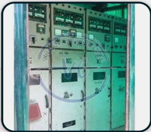
Electrical Control Panel
