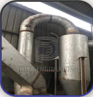
Dust Collection Duct
